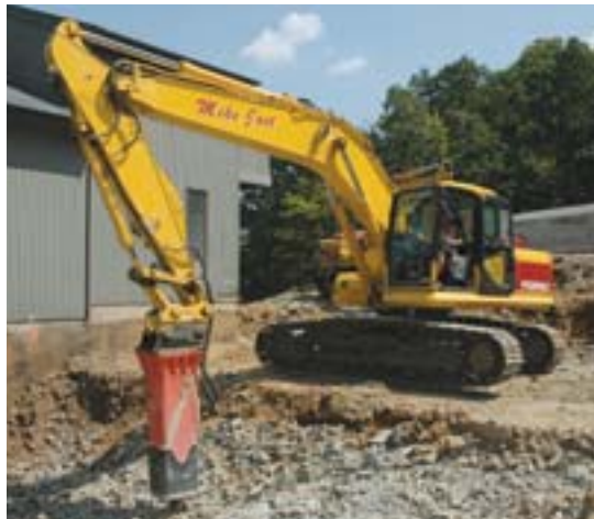
Operator Steve Feaman uses this Komatsu PC200LC-7 excavator equipped with a Stanley MB50EX hammer to break ledge for a swimming pool.
