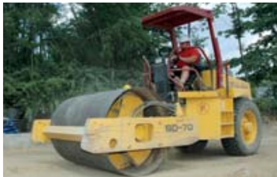
Using an Ingersoll-Rand SD-70 vibratory soil compactor, Operator Bob Mendell prepares an area for a new parking lot for an Upper Saddle River, N.J., customer.
