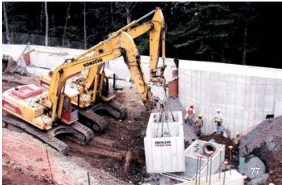
Mike Jost Excavating uses tandem Komatsu excavators (a PC220-6 and a PC300-6) to set trench boxes at Colonial Road School in Franklin Lakes, N.J.
